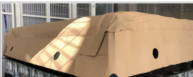
Fig. 20: Deformed inverted tray
